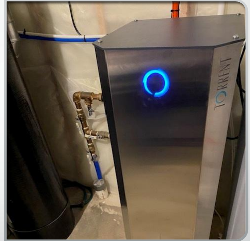
Torrent reverse osmosis filter and pump system.
