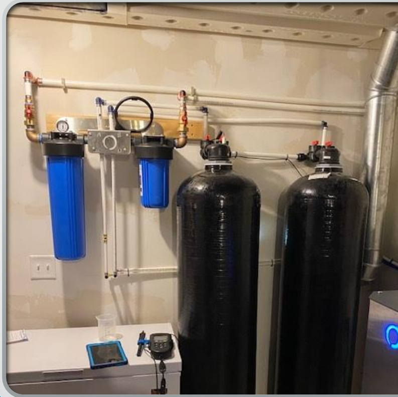
Part of the whole house system: Filter, remineralization, and storage tanks.
